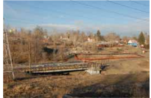
RTD West Corridor Light Rail Bridge Just West of Perry Under Construction on Jan. 24, 2009
